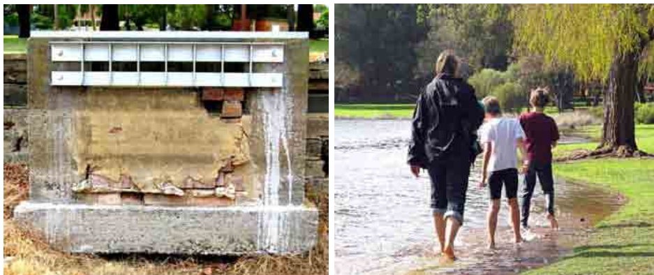
Left , new outlet grille installed early in 2011 makes it impossible to measure or observe the flow. The badly deteriorating brickwork was not repaired. Right , flooding over footpath, August 2011
