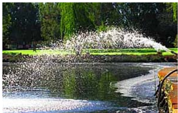
A pump aerates water at Lake Jualbup. It may look good but treating the whole lake at 8 hours/day and 5 days/week would take at least three months.
