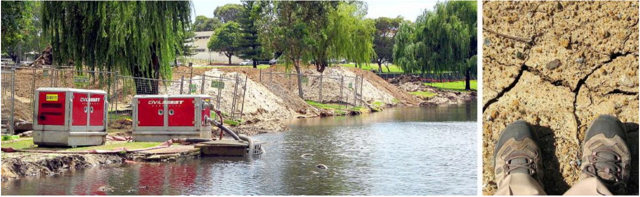
Each pump (red boxes) discharges 50kL a second down the outlet. The mounds in the background are natural clay mix ready for use. Their clay content is confirmed by cracking as it dries after rain.
