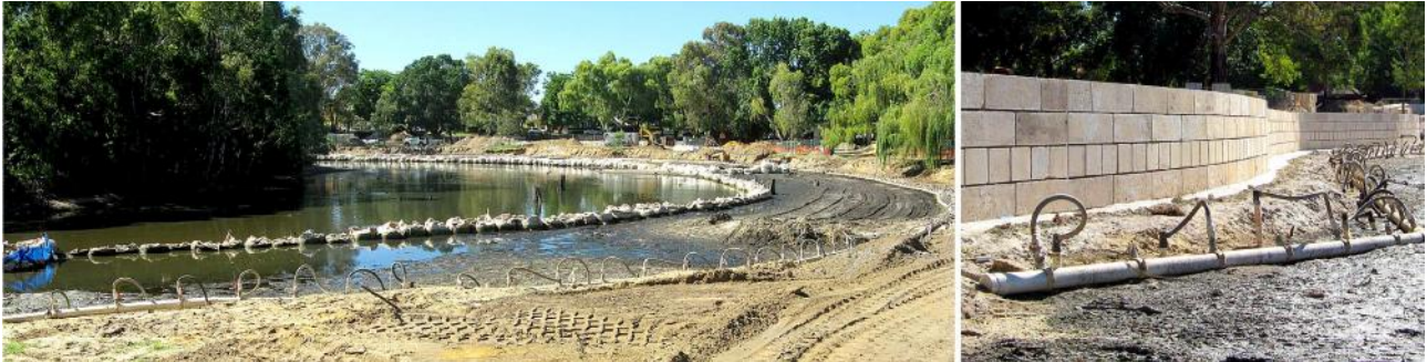
The pumps remove water via pipes to which are attached long spikes driven into the groundwater.
